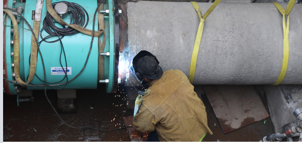
Senior Service Worker Tony Espinoza Jr. welds the new pipe for the effluent line.
