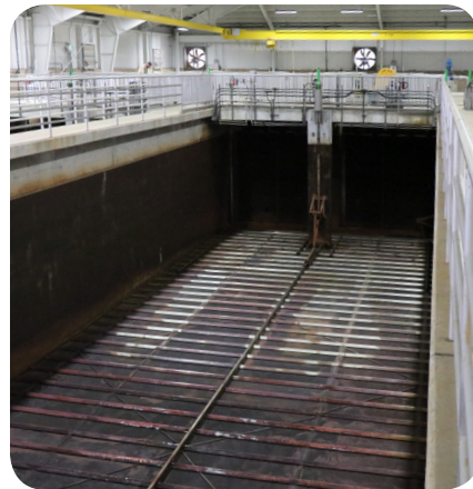
One of the sedimentation basins is drained for cleaning and inspection.
