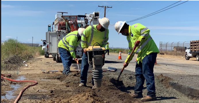
PWD Construction Crew working on 20th Street East and Rancho Vista Boulevard.
