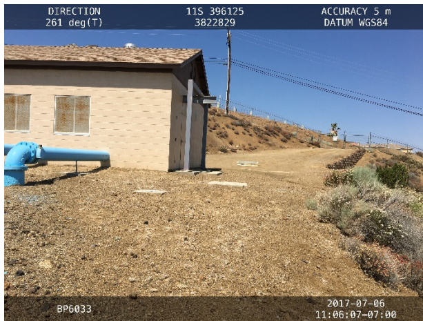
Photo 8. Pump Station FB-02.
