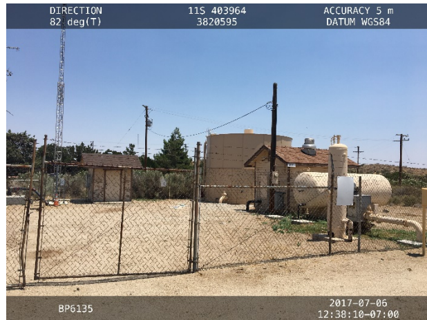
Photo 6. Pump Station EB-01.
