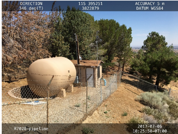
Photo 7. Pump Station FB-01.
