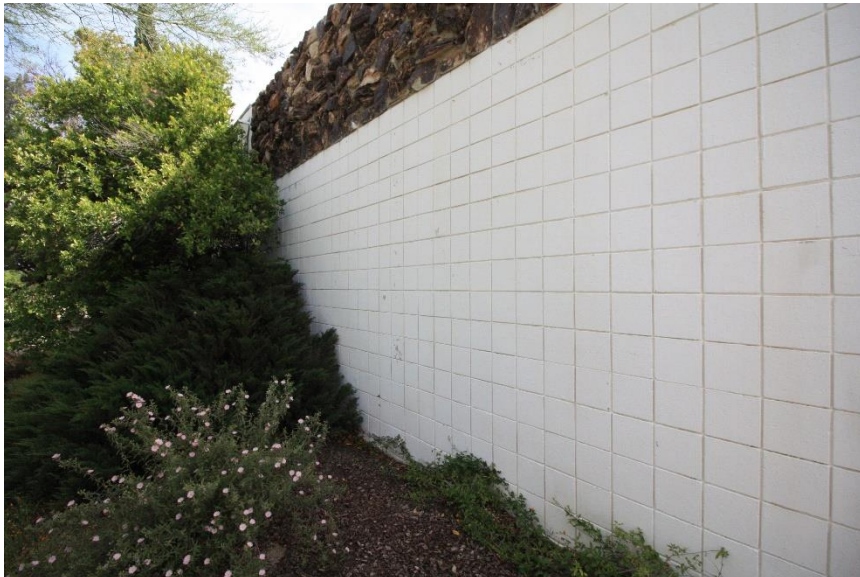
PWD Headquarters, south portion of the west elevation, view to northeast (ESA April 30, 2018)
