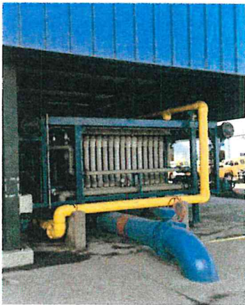
Membrane Filtration System
