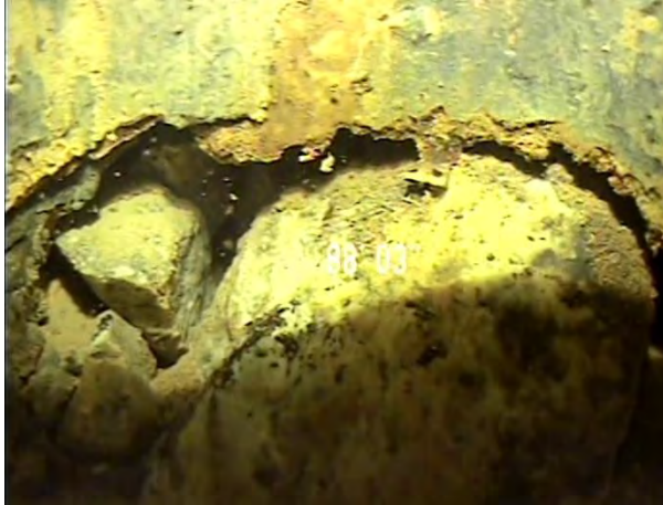
Massive rupture in well screen showing formation cobbles.
