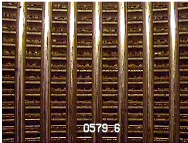
Clean and open well screen with visible gravel material.
