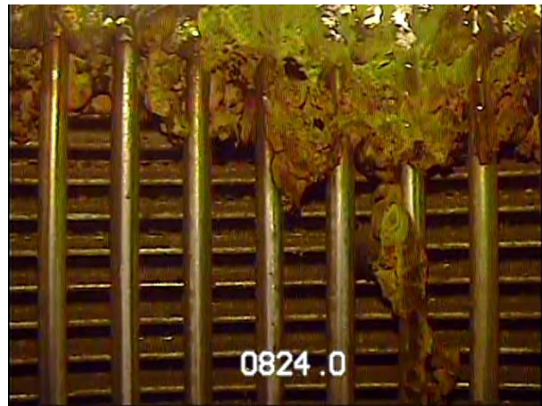
Corrosion byproducts bleeding from blank into well screen.
