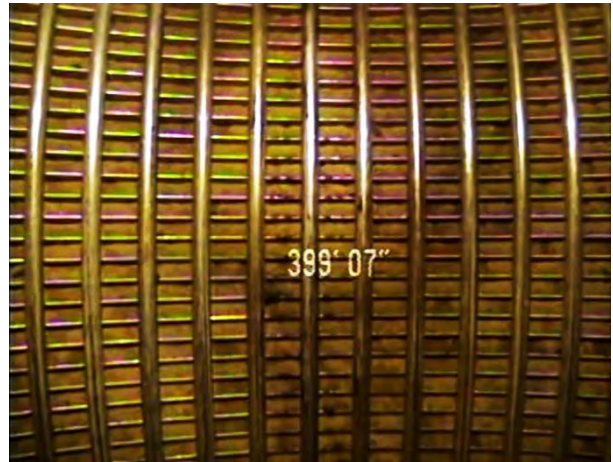
Lower well screen partially clogged with sediment.
