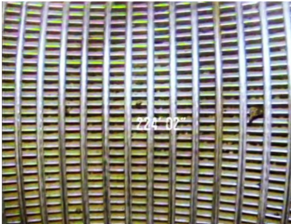
Upper well screen open and in excellent condition.
