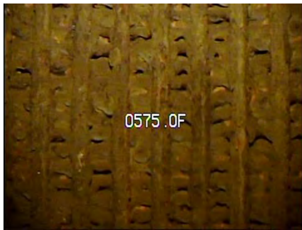
Heavily clogged well screen.
