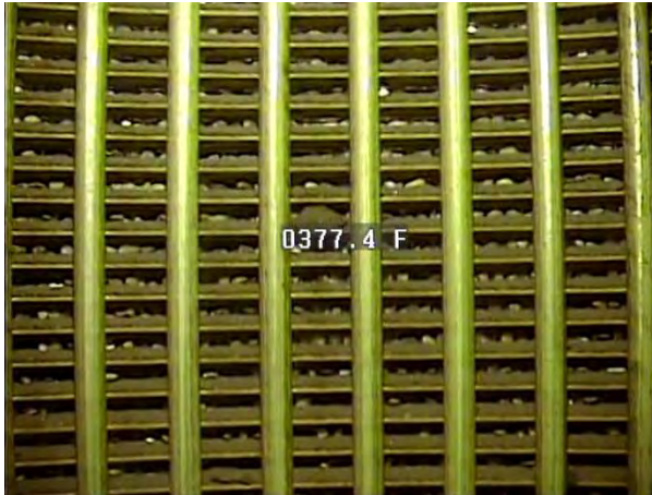
Well screen open and in excellent condition.
