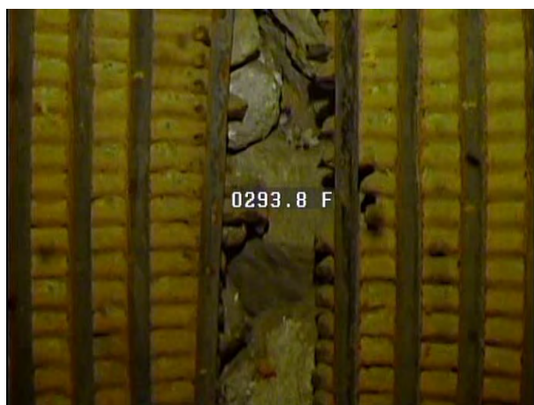
Heavy bacterial growth and severe vertical rupture.
