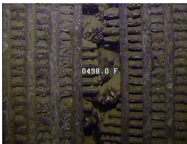
Heavy bacterial growth and severe vertical rupture.
