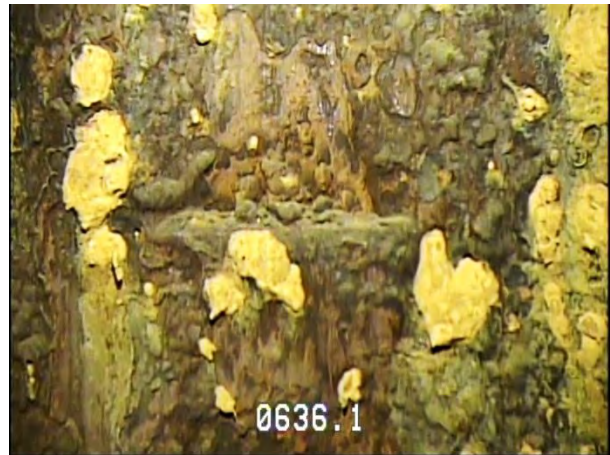
Heavily buildup of bacterial growth on louvered well screen.
