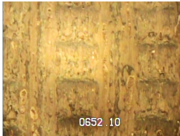
Louvers completely obscured by mineral encrustation.
