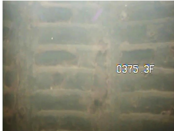
Sediment resting upon the louver shelves.
