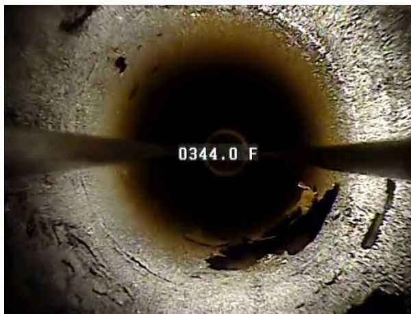
Numerous holes within the 1987 well liner.
