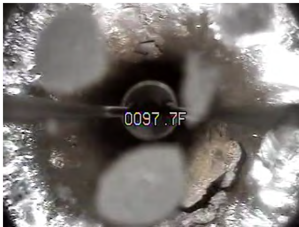
Severe corrosion of blank well liner above water level.
