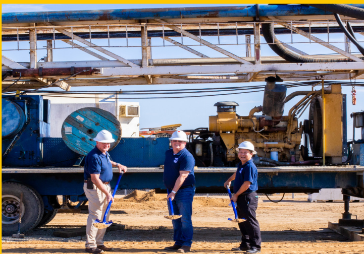
GM Dennis D. LaMoreaux, Engineering Manager Scott Rogers and Assistant GM Adam Ly break ground at Well 36.
