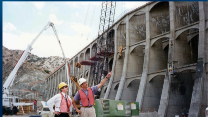
The original facade of the Littlerock Dam was covered with a large roller-compacted concrete buttress in the 1990s.
